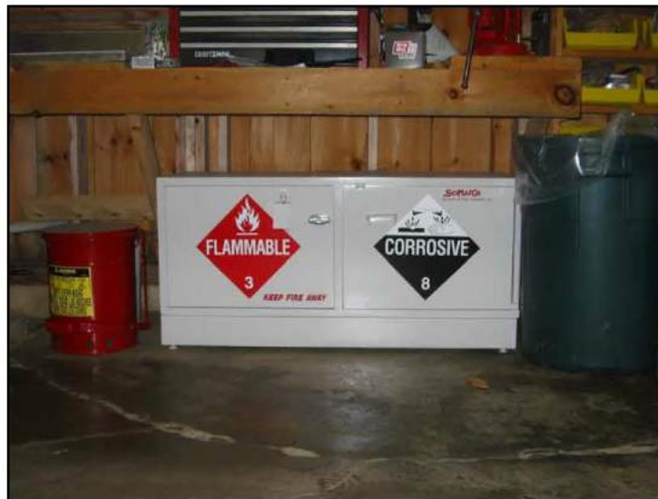
A chemical storage cabinet in a sugarhouse. These cabinets are a great way to store chemicals safely. They minimize the extent of spills, contain small fires and keep chemicals dry, away from incompatible chemicals, food and the public.
